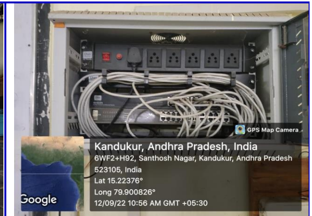
Server Rack-Computer Science Lab-2
